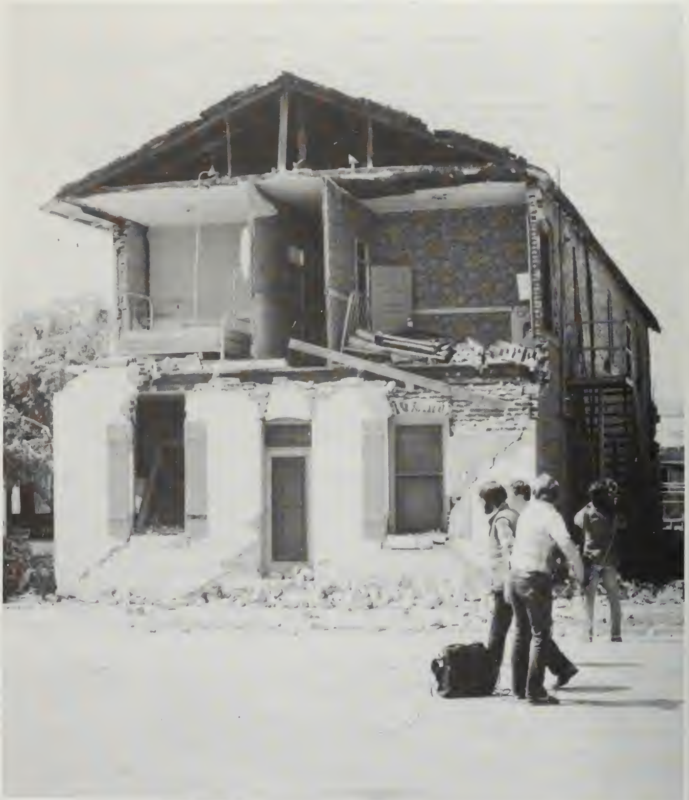
Severe damage to an old motel caused by strong ground shaking during the 1983 Coalinga earthquake. Such damage is very typical for unreinforced masonry structures (URM). Recent California law requires local government to prepare an inventory of URM's within their jurisdiction in order to help identify those buildings that are in greatest need of seismic retrofitting. Delineation of seismic hazards zones can help prioritize URM hazard mitigation programs. Photo by Charles Real.
